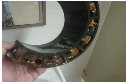
Fouled internals of Turbidity Meter
