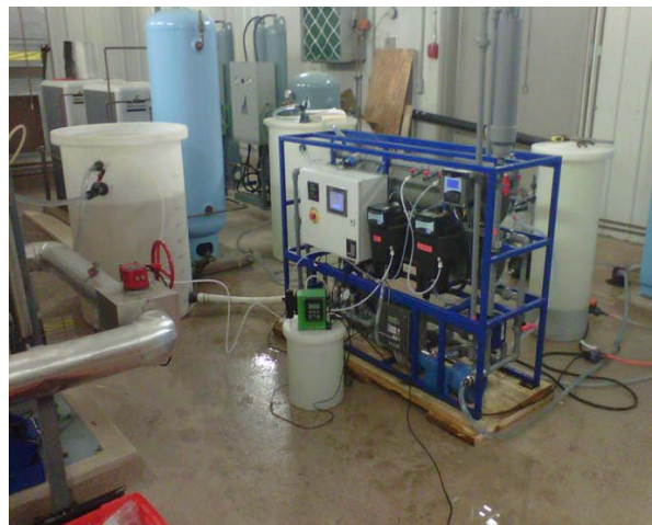
FYNE Membrane Pilot System Setup in former Ozonation Room in WTP
